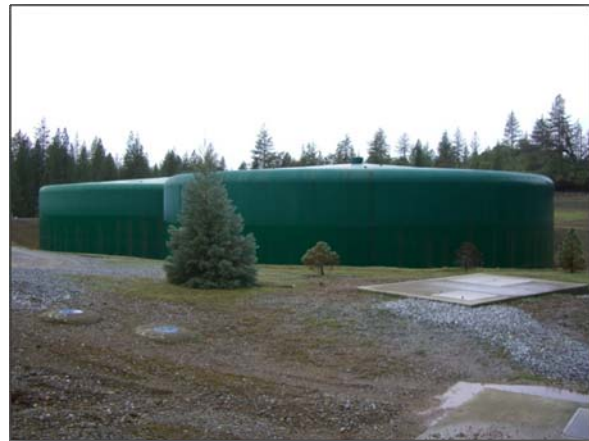
Photo 9 – Tanks and Pressure Reducing Station at Reservoir 7
