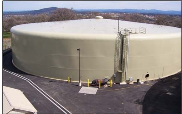
Photo 3 – One of Bass Lake Tanks
