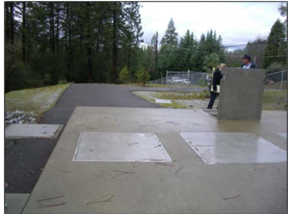
Photo 10 – DSM Pressure Reducing Station No.1
